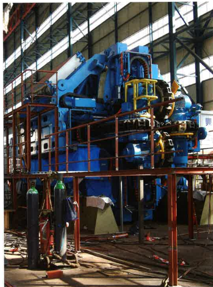
The 200 ton tensioner ensures the pipe is lowered from the ship in a controlled manner
